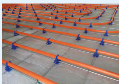
Exemple of heating system
